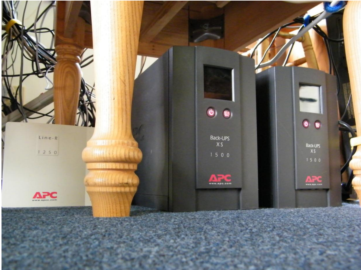
APC Power Conditioner & Uninterruptable Power Supplies in Author's Office
